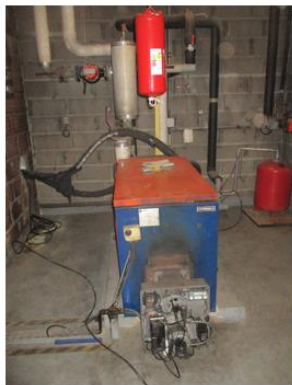
Origin : Fuel Boiler
